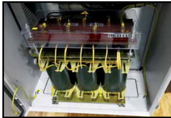
Incoming power transformer
